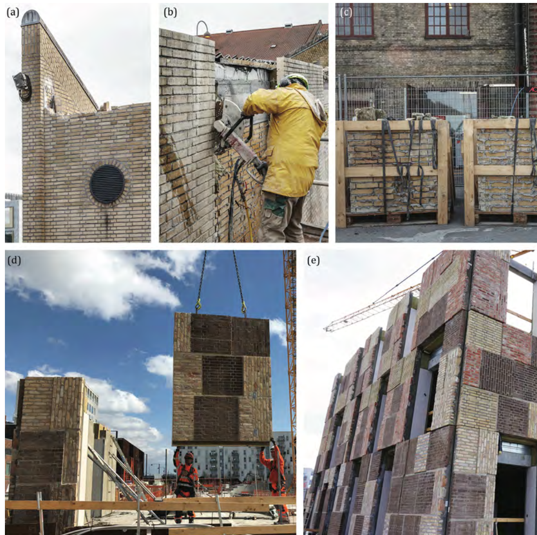
Fig. 02 - Creation of reclaimed masonry modules, by cutting (b) whole parts of brick works (a), stocking the recovered components (c), turned into industrialized panels for the construction of the façades (d) of the residential complex The Resource Rows (e). Pictures: © Lendager Architekt.
