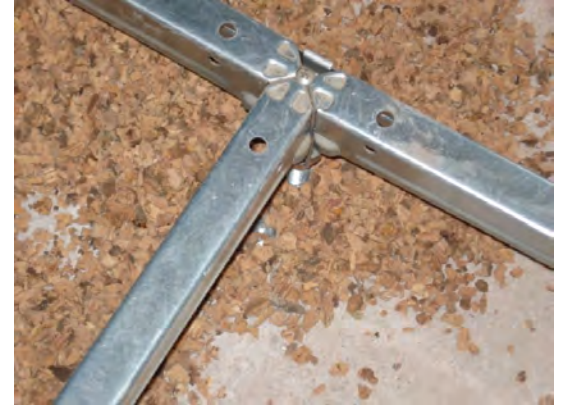
Fig. 10 - Savno' s building, Conegliano, 2008. Floor insulation made of cork. Available at: www.savnoservizi.it
