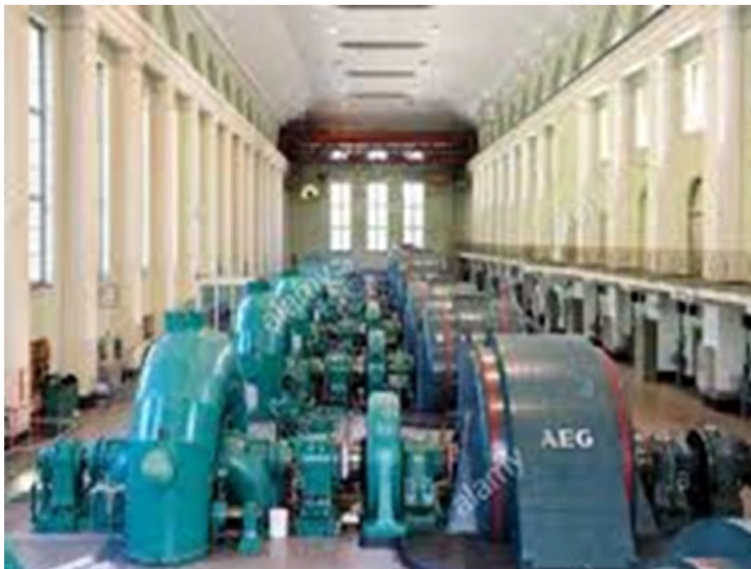
Fig. 11 - Turbine hall of Walchensee Hydroelectric Power Station, Kochel, Upper Bavaria, Bavaria.
