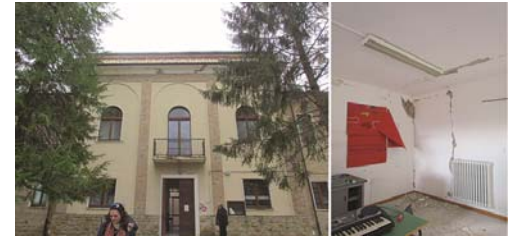
Fig. 4. Gualdo, the old school "Romolo Murri" after the earthquake: the main façade and a classroom (photo credits: R. Marmorì, 16/12/2016).
